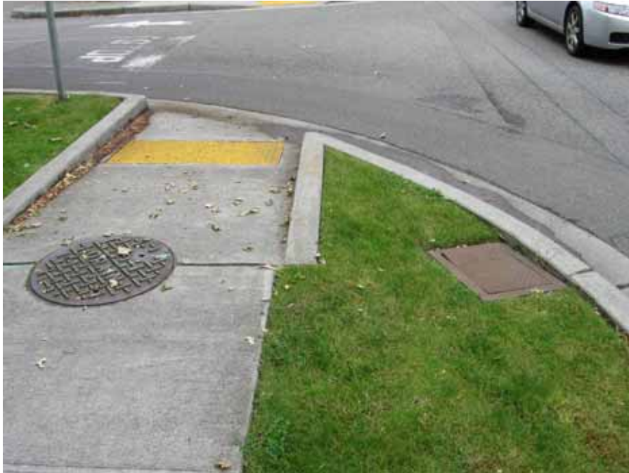
Photo #1—Critical conveyance invert location #4, Southeast corner of NE 24 th Street and 151 st Place NE. Facing west.
