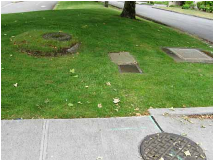
Photo #2—Critical conveyance invert location #4, Southeast corner of NE 24 th Street and 151 st Place NE. Facing south.
